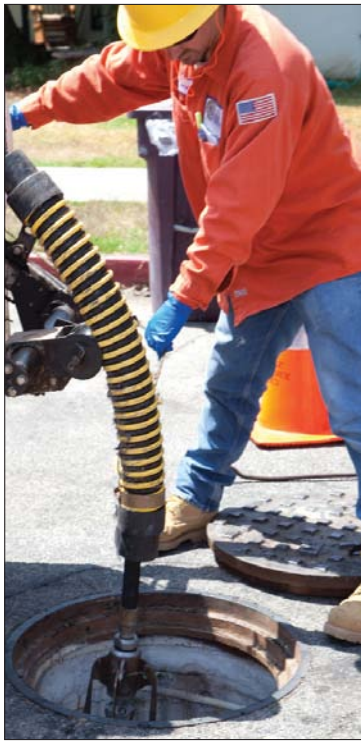
Wastewater maintenance worker Jason Badgley lowers a cleaning nozzle into a manhole.
