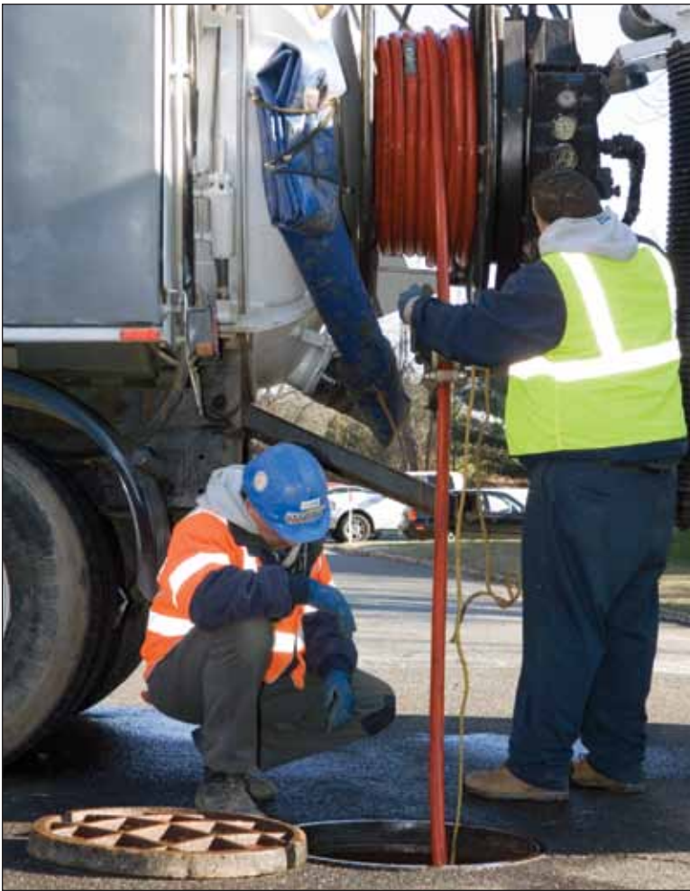
Supervisor Ray Rios and operator Darryl Stephens operate a combination truck on a sewer maintenance job.
