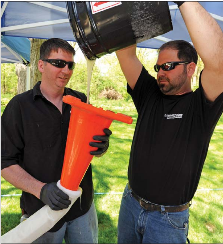
Clayton Holland and Paul Rickert saturate a CIPP liner with resin before putting it into the inversion tank on a residential repair.
