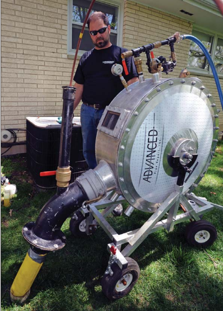
Paul Rickert uses the inversion tank to complete a CIPP lining job using technology from LMK Enterprises Inc.
