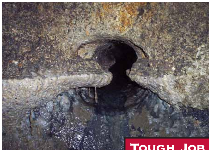
The 8-inch sewer main had no invert and was occluded with grease, lime deposits, rust buildup, and corrosion.
