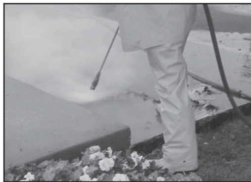
Using the StoneAge Barracuda to remove an elastomeric membrane from a walkway.
